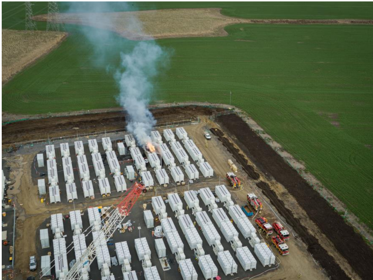
Figure 4 Victoria Big Battery fire incident [47]
