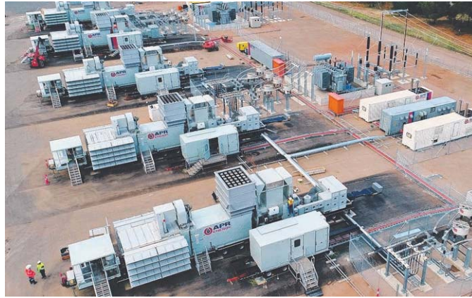
The diesel generators at the former Holden factory
